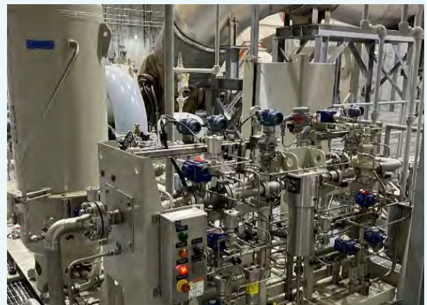
National Fuel's DGS system reduces methane emissions from their compressor station.
