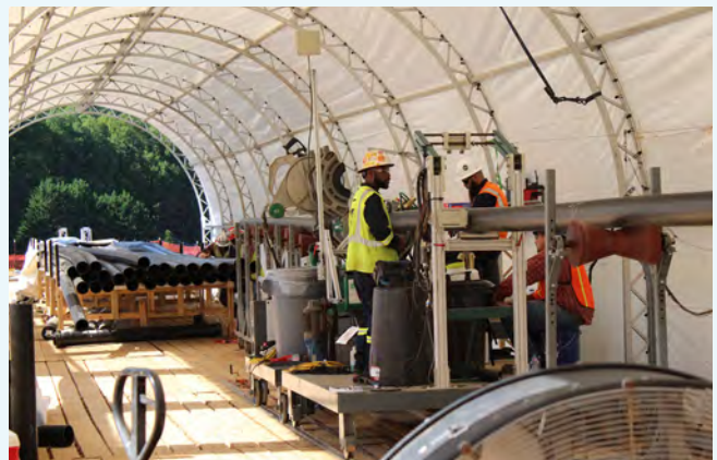
Enbridge workers produce the company's innovative liner product at a Smartpipe mobile factory.
