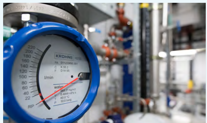
Above: The Markham, ON, Power-to-Gas facility produces clean hydrogen that's injected into the Enbridge Gas distribution network.
