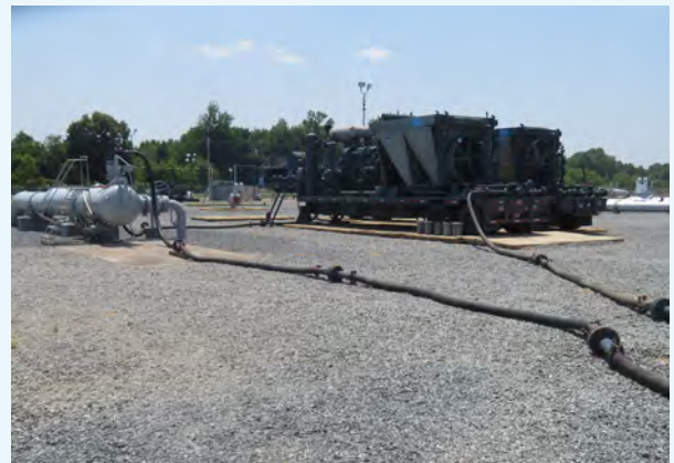
Mobile compression units at a TC Energy compressor station.
