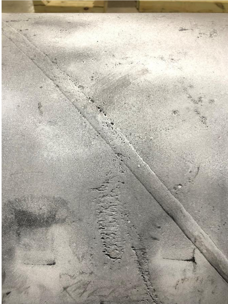
Figure I-3. Example of corrosion and SCC near a spiral weld
