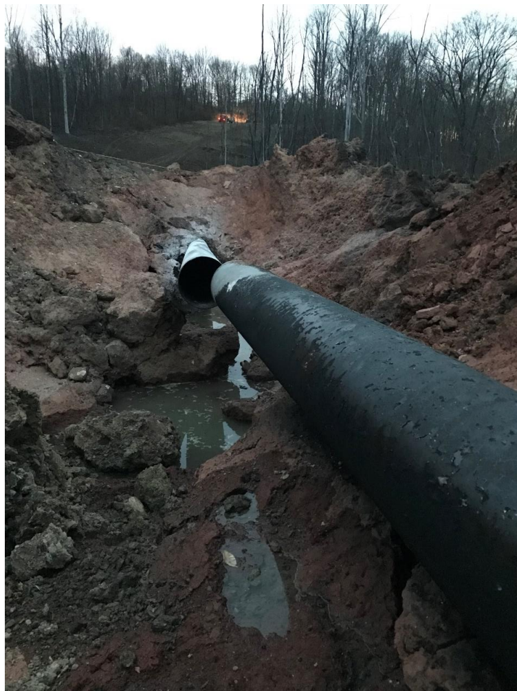
Figure C-9. In-service failure of a girth weld with weld strength undermatching
