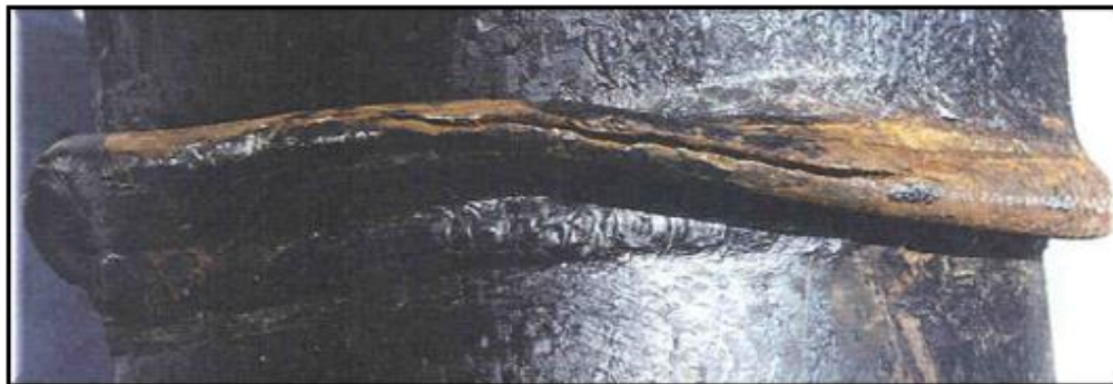
Figure C-3. Wrinkle formation near a girth weld and the resulting cracking of pipe wall at the apex of the wrinkle
