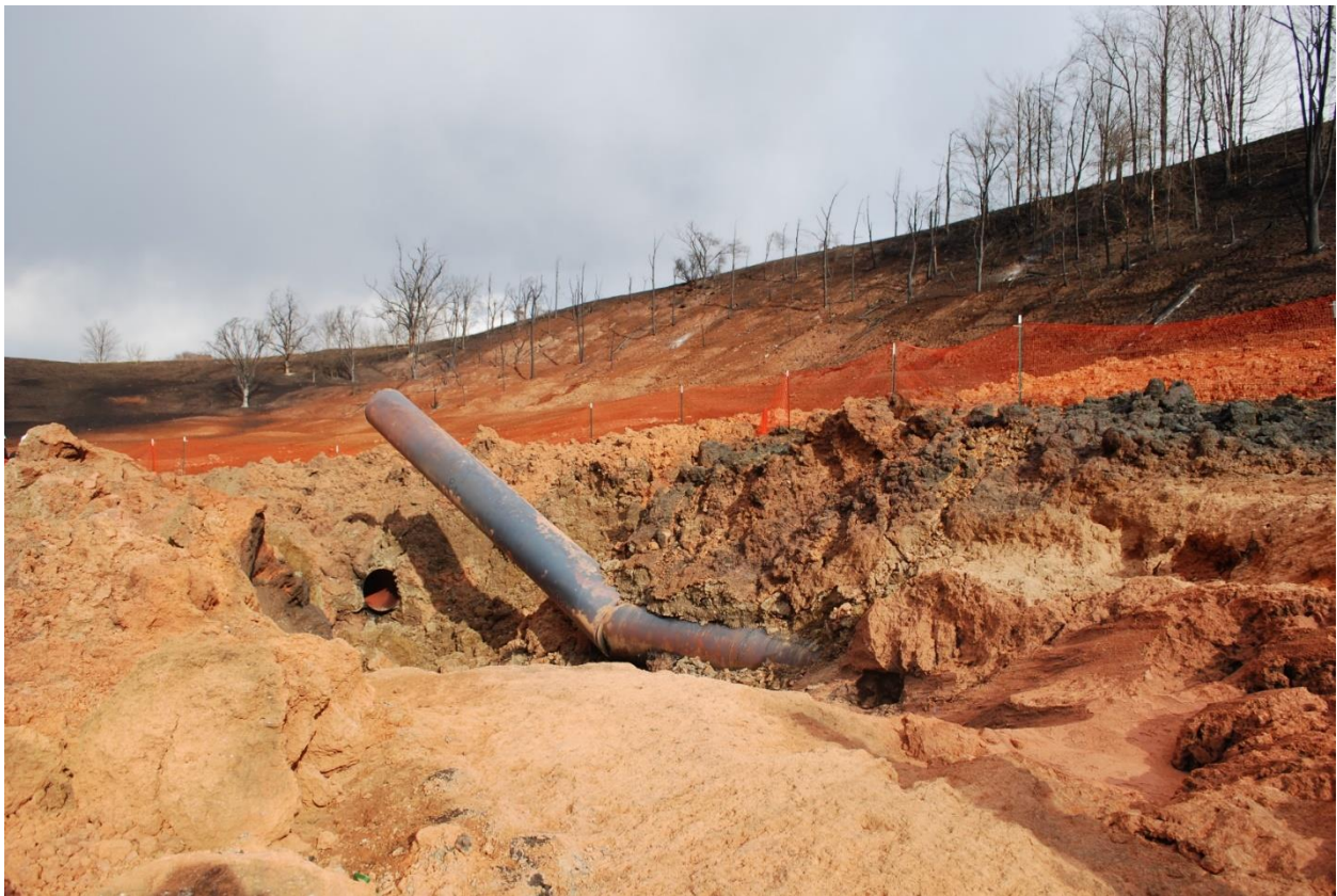
Figure C-6. Failure of a girth weld of a vintage pipeline at low strain due to weld flaws
