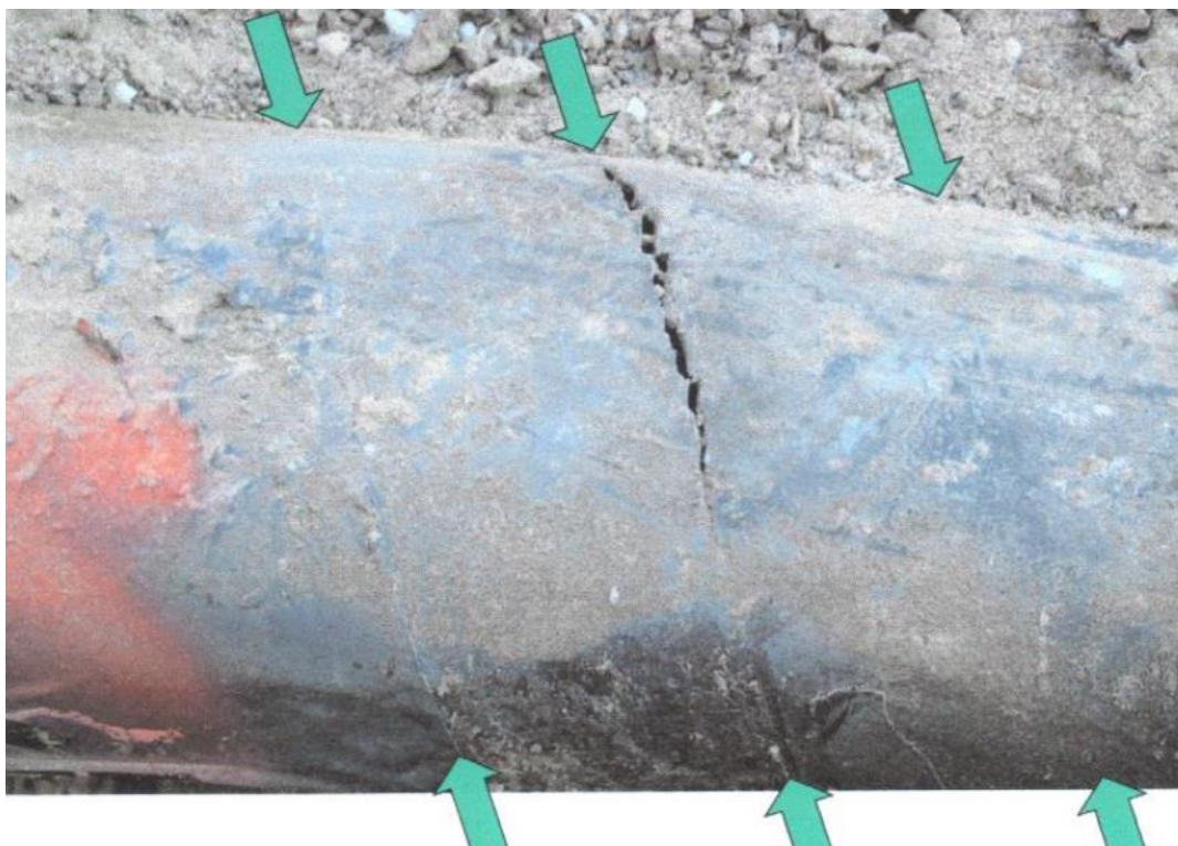
Figure I-2. Example of a S-SCC aligned with tape coating that resulted in a leak
