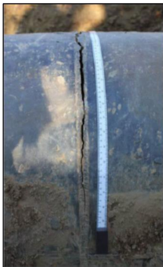
Figure C-1. Example of a girth weld failure due to longitudinal stress/strain
